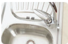
Kitchen Drain Pipes
